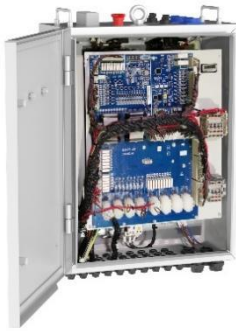
Main control Cabinet
